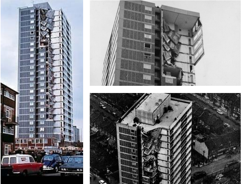
Figure 2-1. Collapse of Ronan Point Building, London, UK (1968) 4
