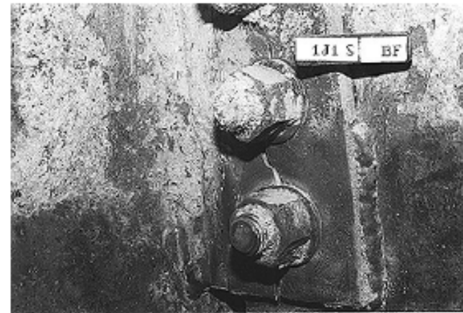
Vertical Fracture through Beam Shear Plate Connection
