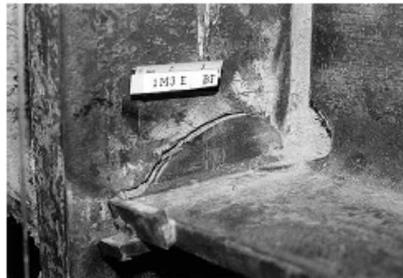
b. Column Flange "Divot" Fracture
