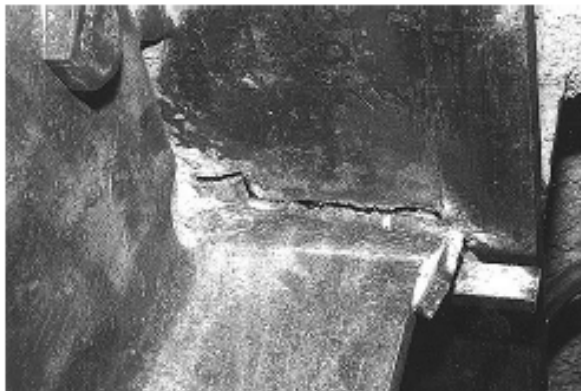
a. Fracture at Fused Zone
