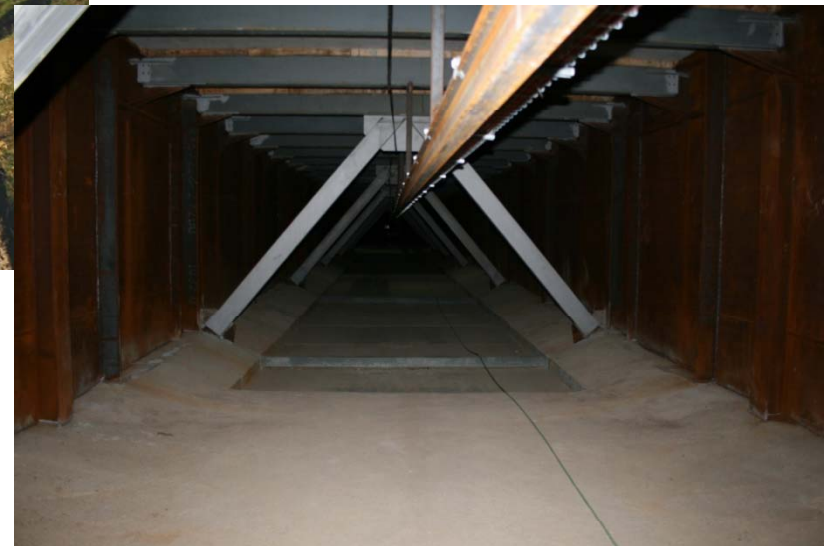
Example of the first Spanish High Speed Railway Viaduct with double composite action
