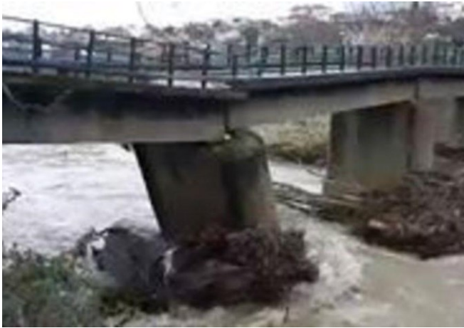
Flash floods on 1 February 2015 Collapse of bridge in Arta, Greece
