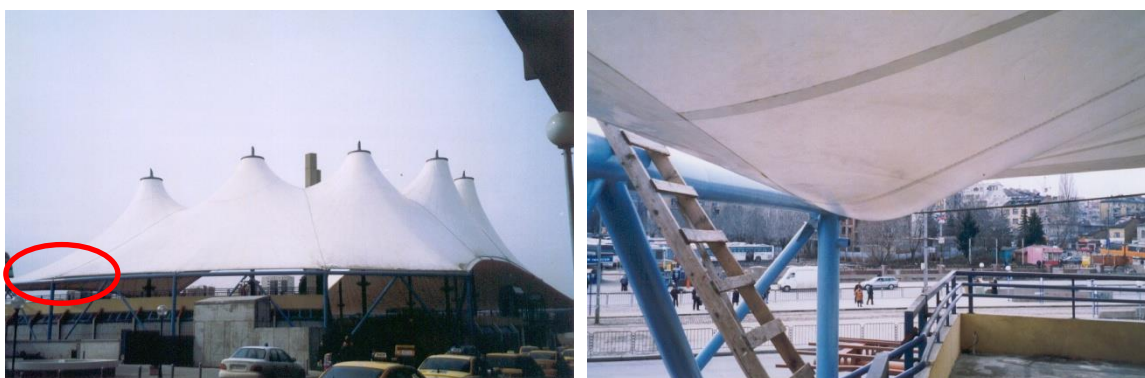
Figure 7-1 Ponding at the corner of conic structures caused by rain load in combination with rotating of the pylons (kinematics displacement) of the supporting structure, Central Railway Station Square, Sofia [© V. Tanev]
