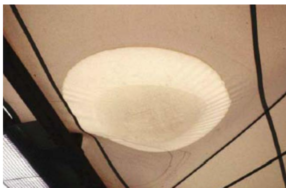
Figure 1-13 Ponding [© J. Llorens]
