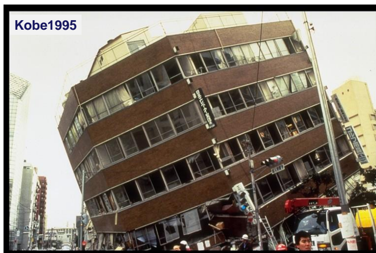
Fig. 4.5.1 Example of damages to a building caused by liquefaction of the foundation soil
