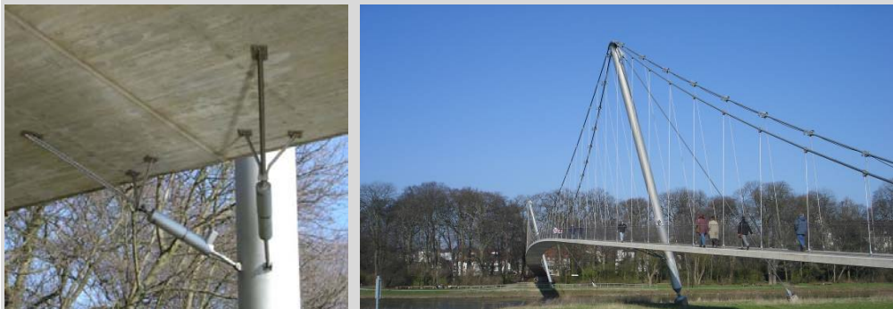
Figure 6-2: Viscous dampers installed at Minden footbridge (Germany)
