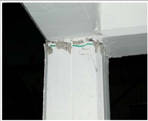
Visible damage after the 0.20g PGA test
