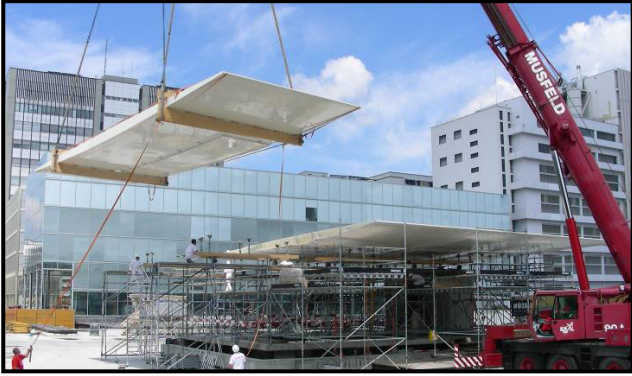
Novartis Campus Entrance Building, Switzerland. Lightweight GFRP cell-core sandwich roof on load-bearing glass envelop. Dimensions 21.6 m x 18.5 m. Designer: prof. T. Keller, 2006.
