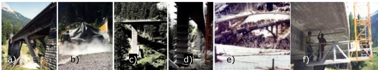
Figure 7.2 Assessment and retrofitting of a series of existing prestressed concrete road bridges of an alpine transit highway [images a) and b) © European Union, 2015]
