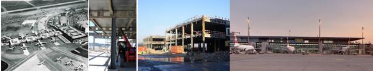
Figure 7.8 Assessment, reintegration, and upgrading of an existing airport building respecting severe restrictions for logistics and construction works due to the tarmac traffic [Left image © European Union, 2015]
